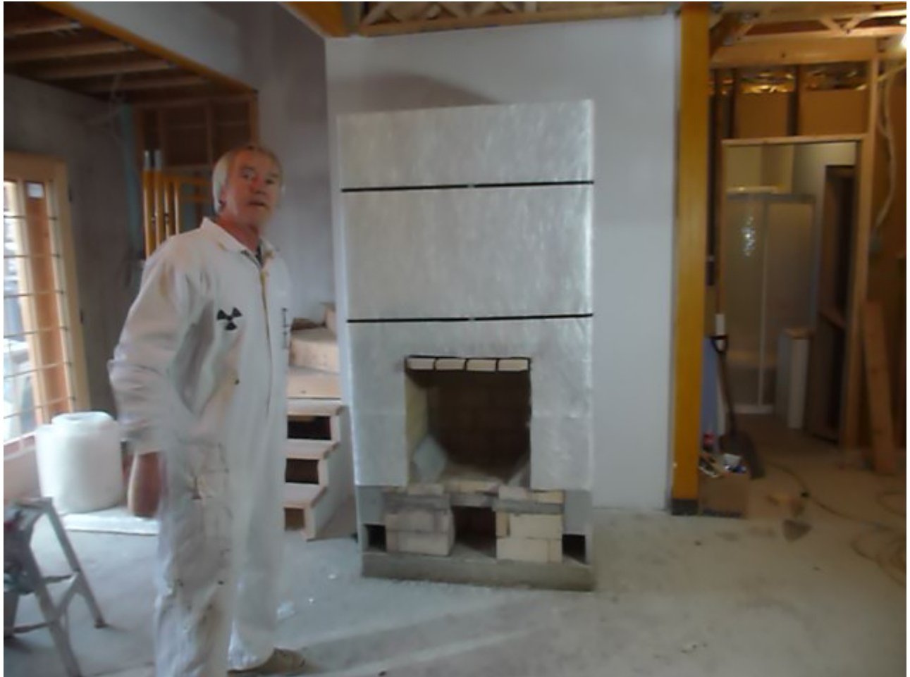
Heater core with fiberglass matt slip joint installed. Ready for facing. This one does not have an oven.
